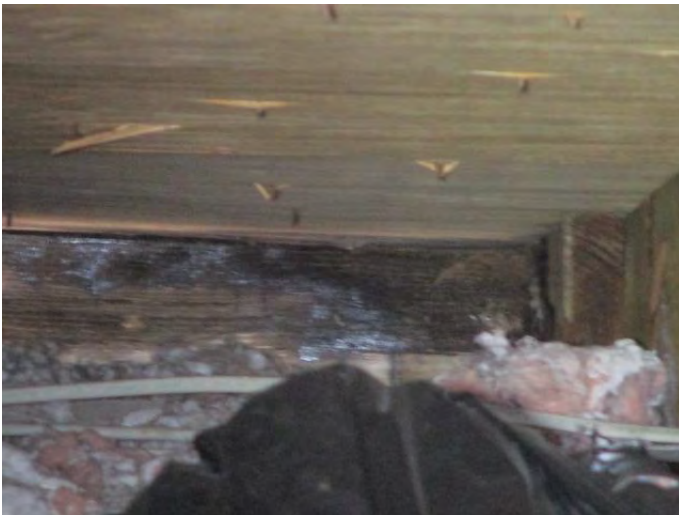
Moisture penetration roof decking attic
