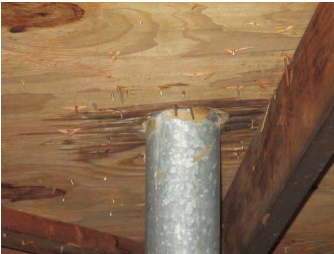
Moisture penetration roof decking
