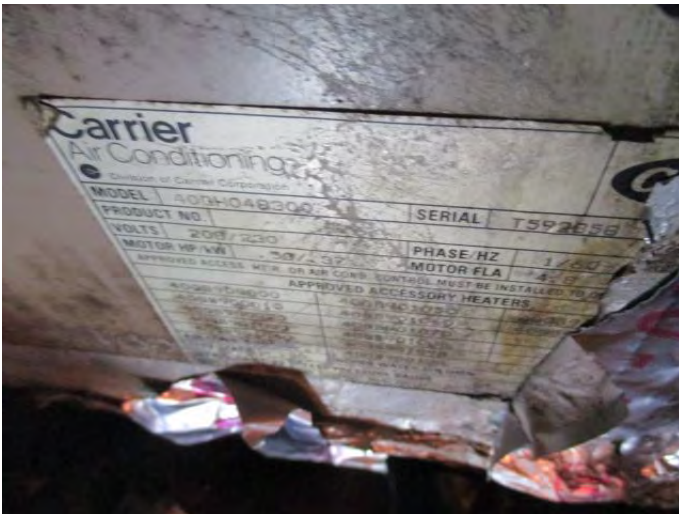
Rust air handler
