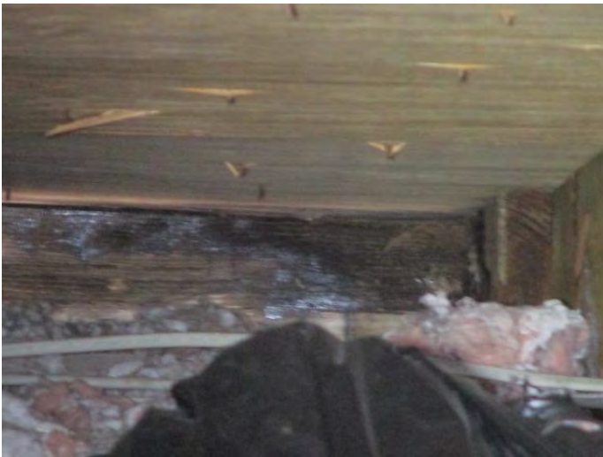
Moisture penetration roof decking attic
