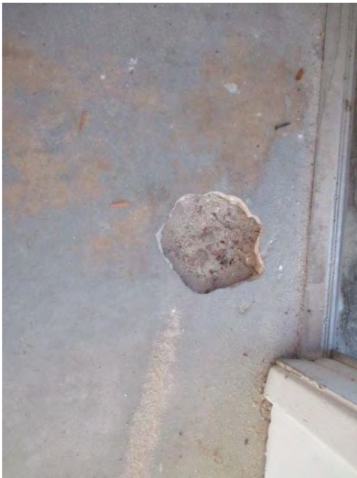
Damaged garage floor
