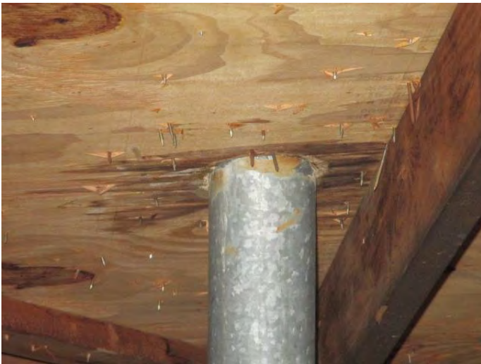
Moisture penetration roof decking
